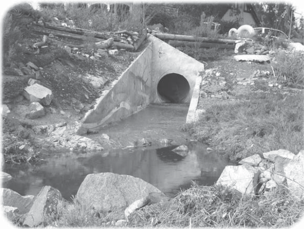
A storm drain outlet which flows unfiltered directly into a local stream.
