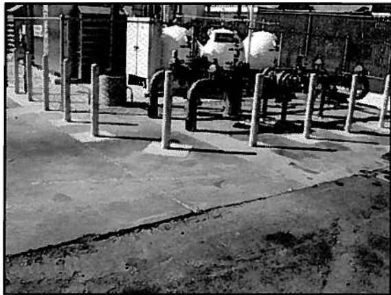
Photograph 3: Example of bollards surrounding CNG Equipment Area
