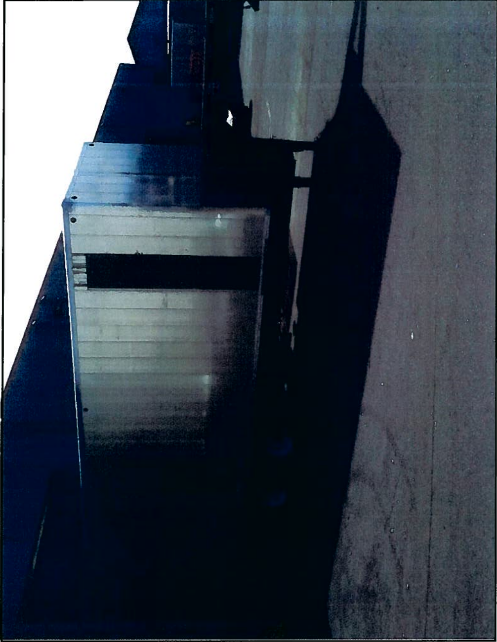
Temporary CNG Trailer
