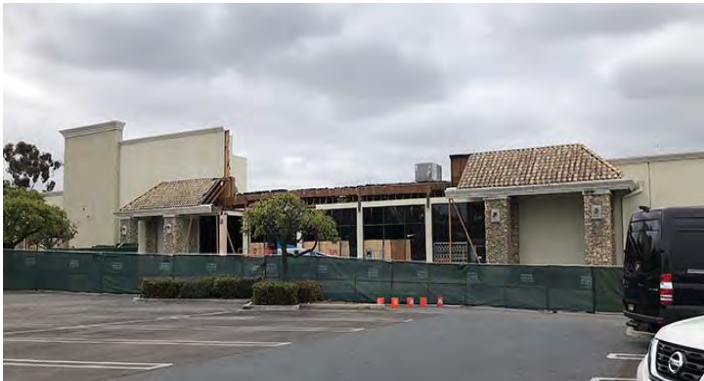
Hobby Lobby has started tenant improvements on a 60,000 sq. ft. building at 3514 Plaza Dr. in the College Plaza shopping center. Hobby Lobby is anticipating a fall 2018 opening.
